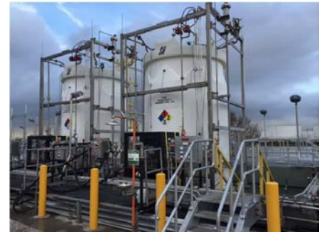
Figure 6 PAA Tote Storage and Pump Skid System
