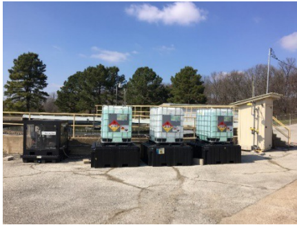
Figure 4 PAA Tote Storage and Pump Skid System
