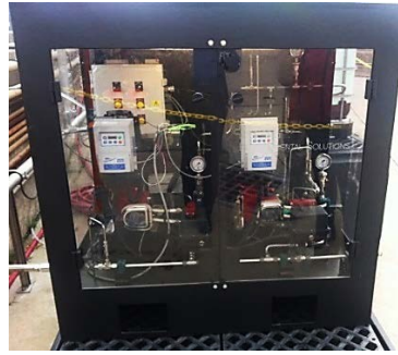
Figure 5 PAA Delivery Pump Skid
